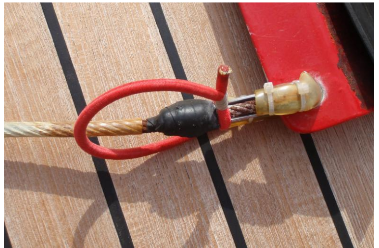
“Soft Tape” used to prevent damage from metal swage with corrosion of wire visible
